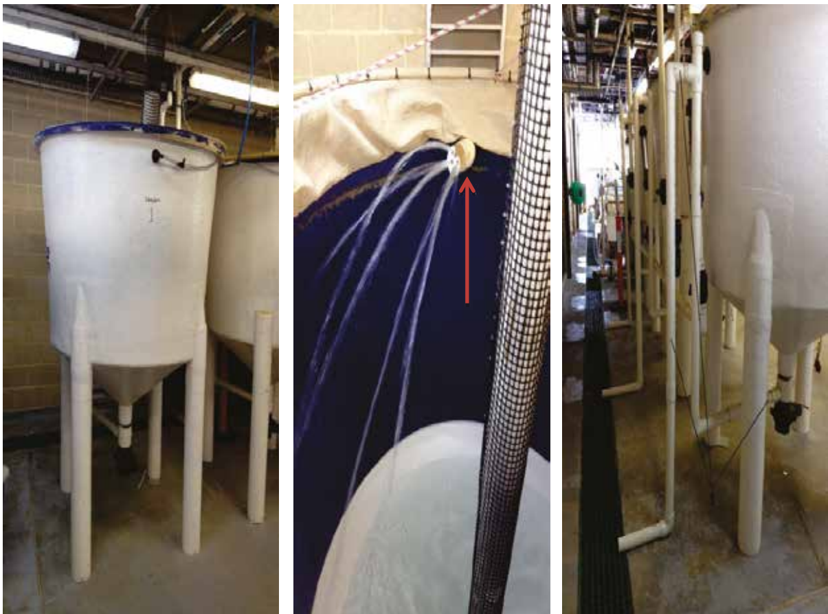
Figure 58. 2300 Lt system and tank components. Red arrow indicates hard plumbed seawater inlet.
